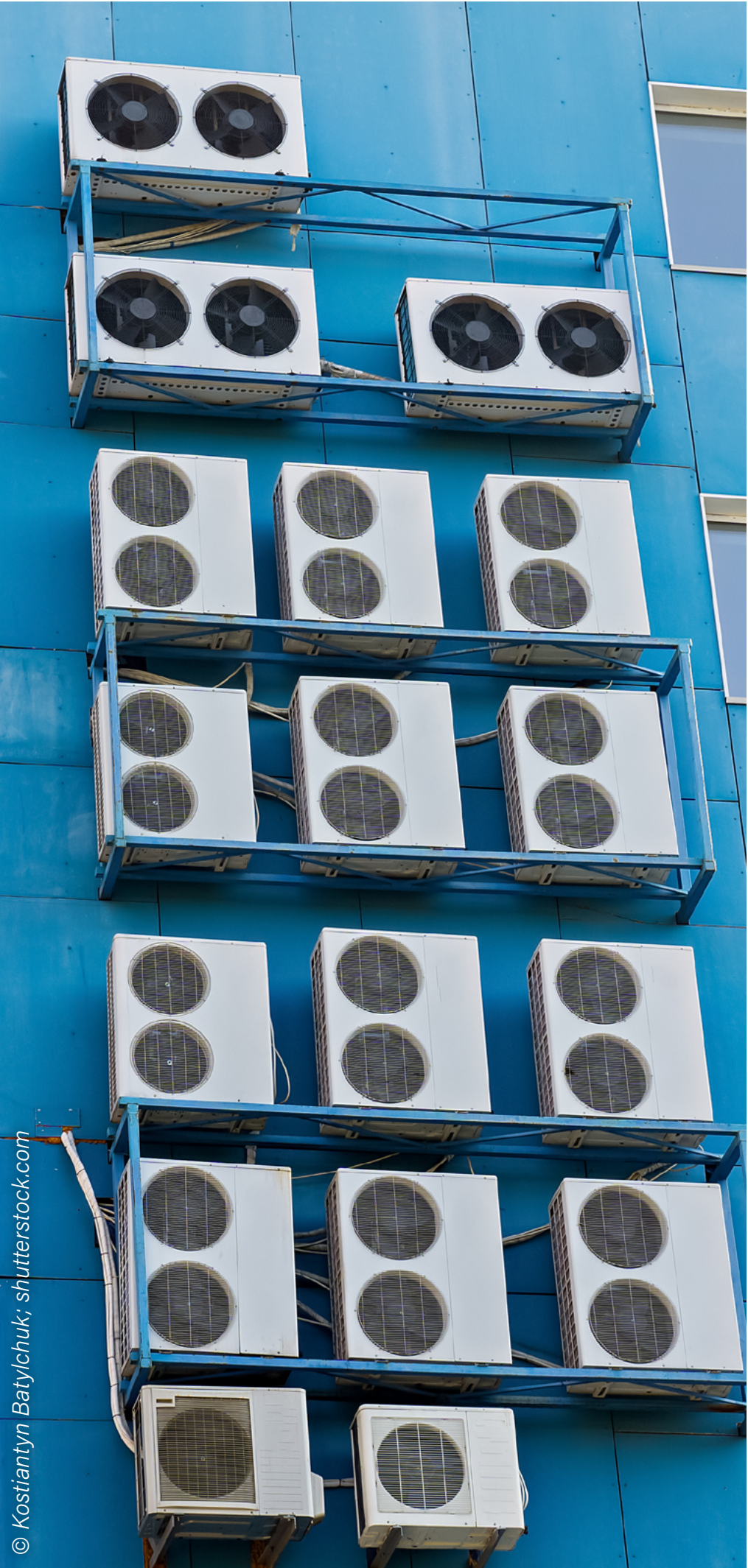
Air conditioning system installed on a building
